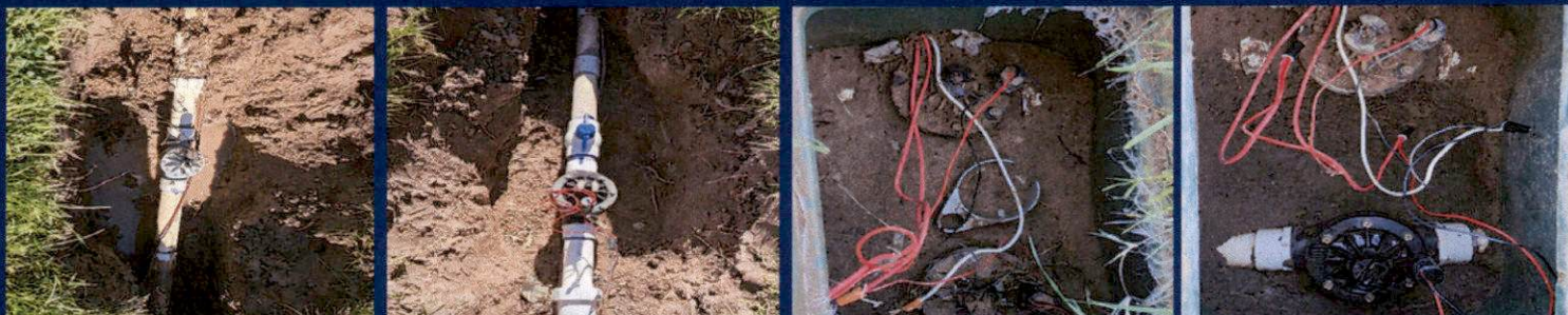
Bienestar Estates (1037 Kennedy Ln.) Bad irrigation valve installed new valve
